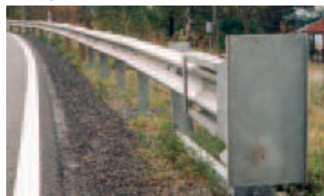
Picture of sharp edged impact absorbing guardrail terminal that can inflict critical injury to a motorcyclist
